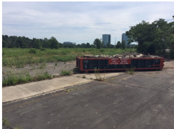
Work at the Purcell preserve is ongoing through the generosity of the BAND Foundation. Pictured is the remnant of old airfield runway we will use as a parking area for visitors and a dumpster filled with concrete debris as part of our restoration work
